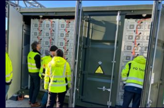
Battery Energy Storage
