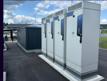
Grid Connection & Charging Infrastructure
